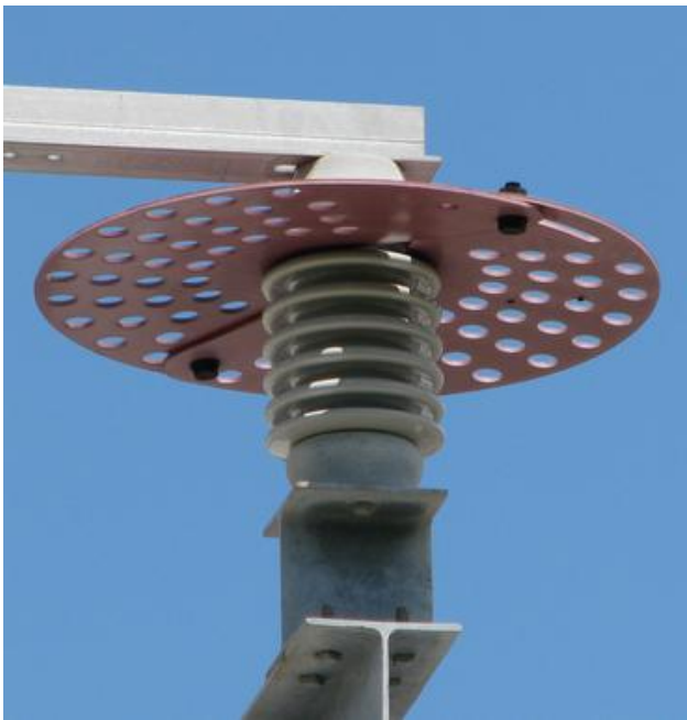
Figure 9 Barrier type WPD mounted too close to the high voltage
