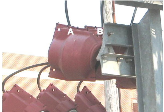
Figure 7 Large arrester cover with poor lead management
