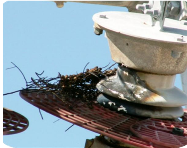
Figure 10 Barrier type WPD compromised by a bird nest
