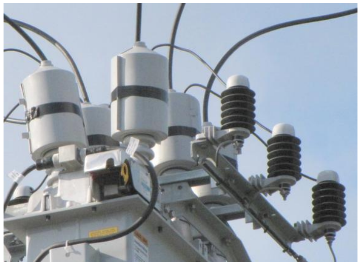
Figure 2: Cover Type Wildlife Protective Devices on the bushings of a recloser and arresters
