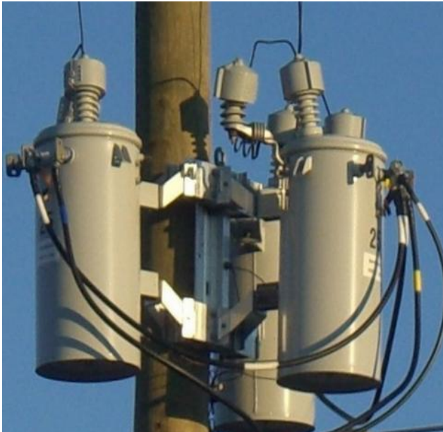
Figure 3: Cover Type Wildlife Protective Devices on Duke Power system.
